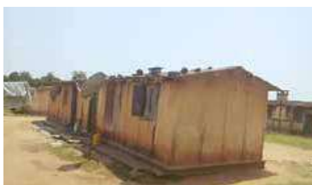
◀ Dilapidated police accommodation at Kitgum Police Station
