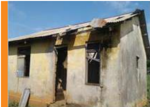
Dilapidated police office at Agwata Police station
