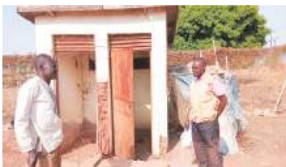
A toilet facility at Padibe West Police Post with one door missing, infringing on privacy. © UHRC
