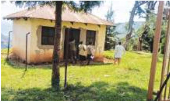
The UHRC inspection team at Rubaya Police Station; the male cell has no ventilation. © UHRC
