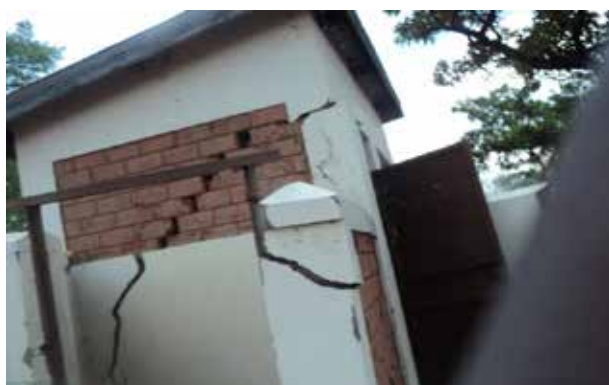
Latrine with a cracked wall at Lapul Police Post in Pader District
