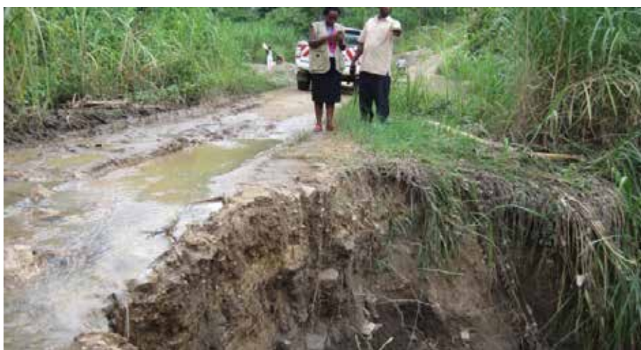
Access road from Kikyo HC IV to Bundibugyo town affected by rains
