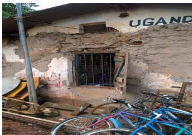
Dilapidated structures at Kitoro Police Station
